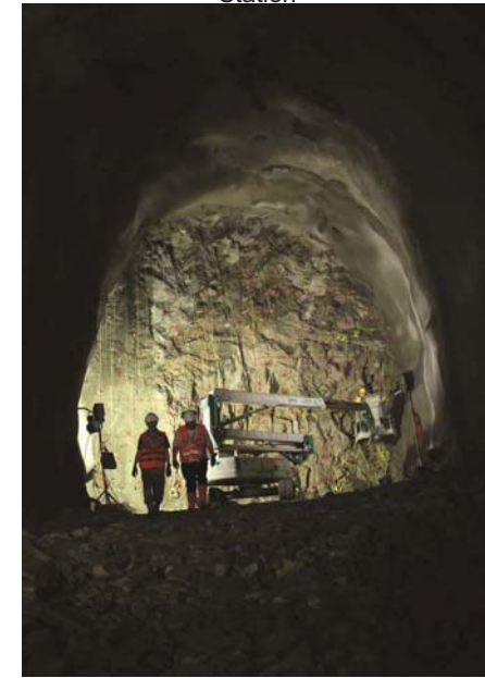
Drill and Blast Tunnel for future Shatin to Central Link at Admiralty Station
