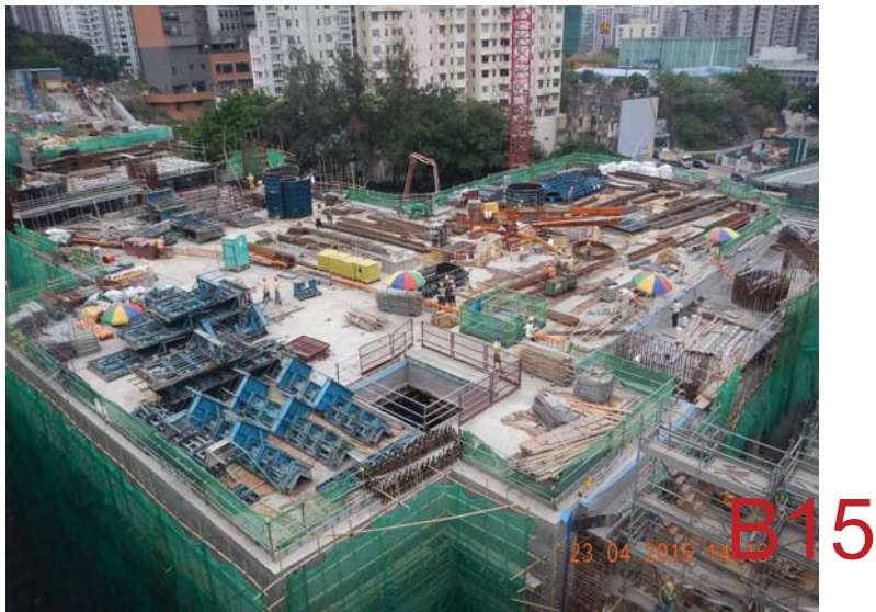
Ho Man Tin Station Construction – Intersection of Kwun Tong Line Extension and SCL EWL
