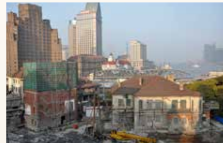
▲ Renovation of historic building to regain the old-look of Shanghai. This photo took in 2009 showed the renovation work for the previous British embassy of Shanghai.
