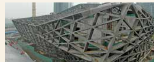
▲ A very challenge example of a special structure, the skeleton frame for the Guangzhou Opera House.
