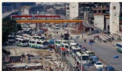
▲ Quite a messy environment working in a road improvement project like this one as seen in Guangzhou in 1998.
