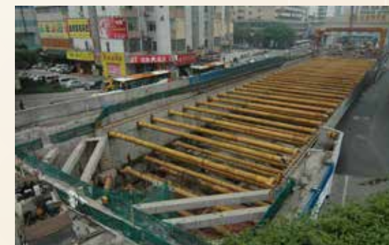
▲ Construction of a section of the Metro Line 5 near Zhujiang New Town. (珠江新城)
