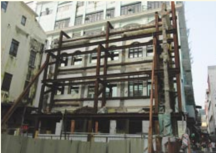
A facade panel being temporarily preserved and supported with rows of shoring frame for a redevelopment project near the Senado Square
